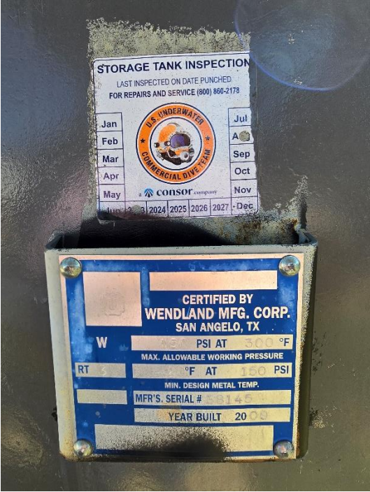
PUMP STATION 2 EXISTING PRESSURE TANK 1 NAMEPLATE
