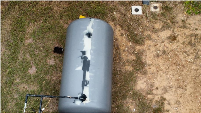
PUMP STATION 2 EXISTING PRESSURE TANK 1 TOP VIEW
