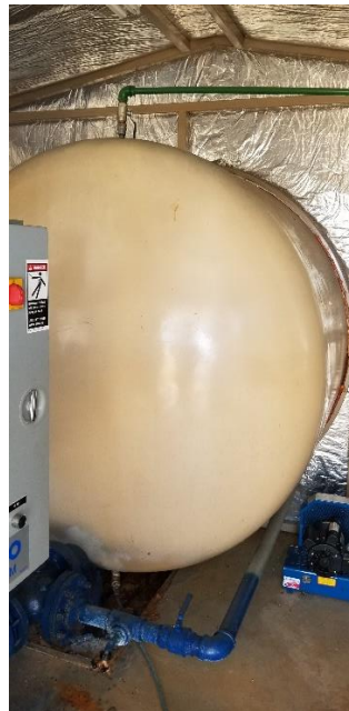
PUMP STATION 3 EXISTING PRESSURE TANK INSIDE BUILDING VIEW
