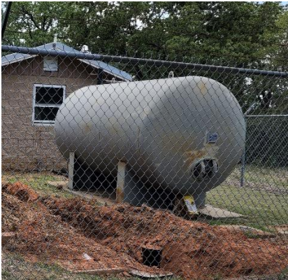
PUMP STATION 2 EXISTING PRESSURE TANK 1 SIDE VIEW
