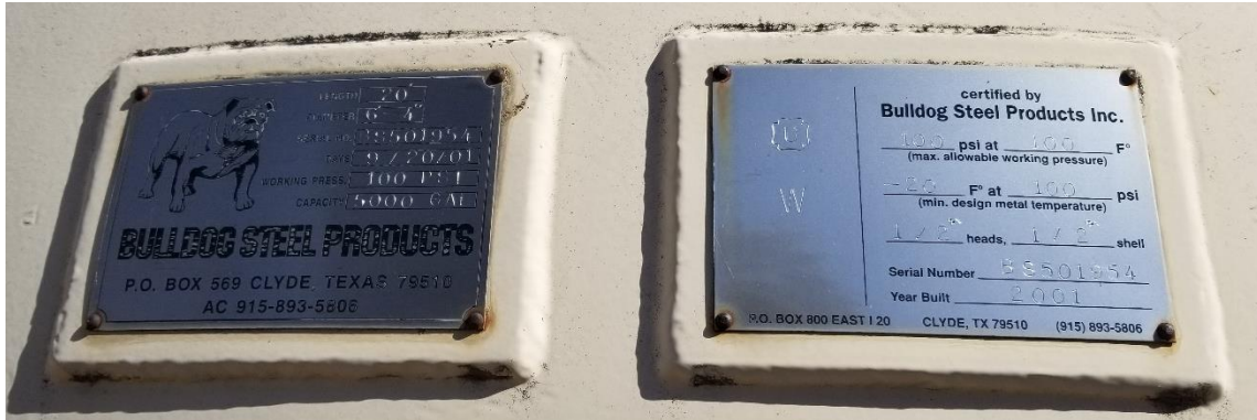
PUMP STATION 3 EXISTING PRESSURE TANK NAMEPLATE
