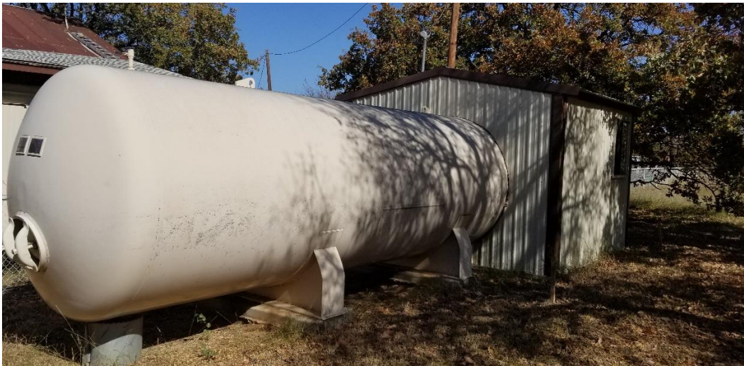
PUMP STATION 3 EXISTING PRESSURE TANK SIDE VIEW
