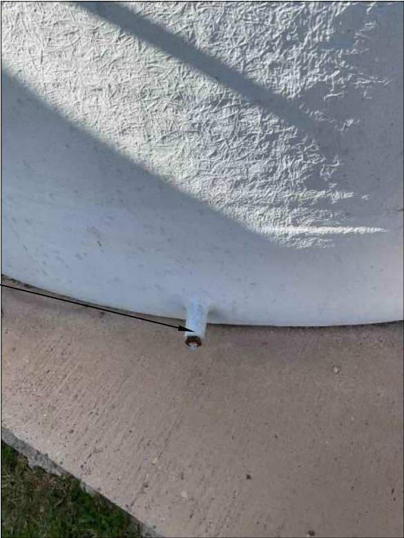
CLOSE UP PHOTO OF GROUND STORAGE TANK 1/4" PLUG
