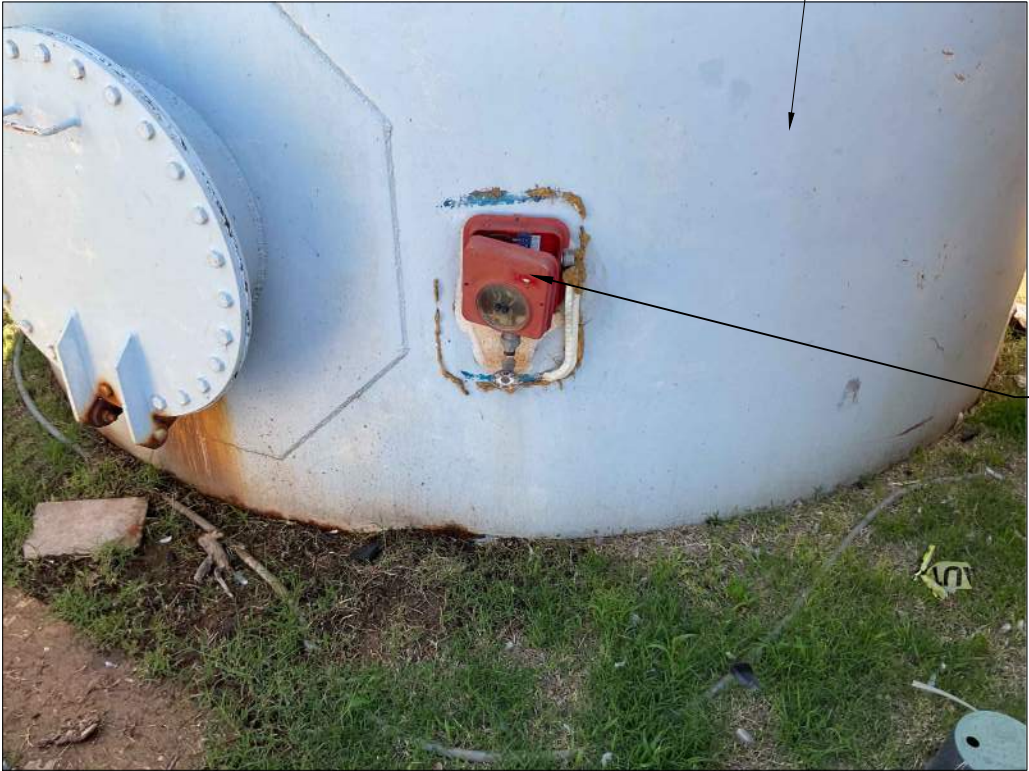
TOWN NORTH ESTATES GROUND STORAGE TANK
